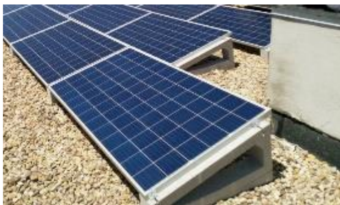
Figure 1. Racking used to support PV panels
