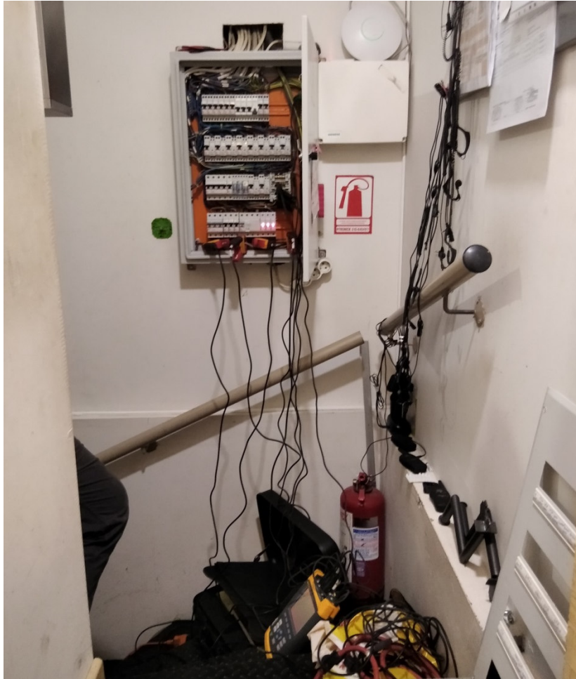
Photo 5: Installed electrical energy measurement system
