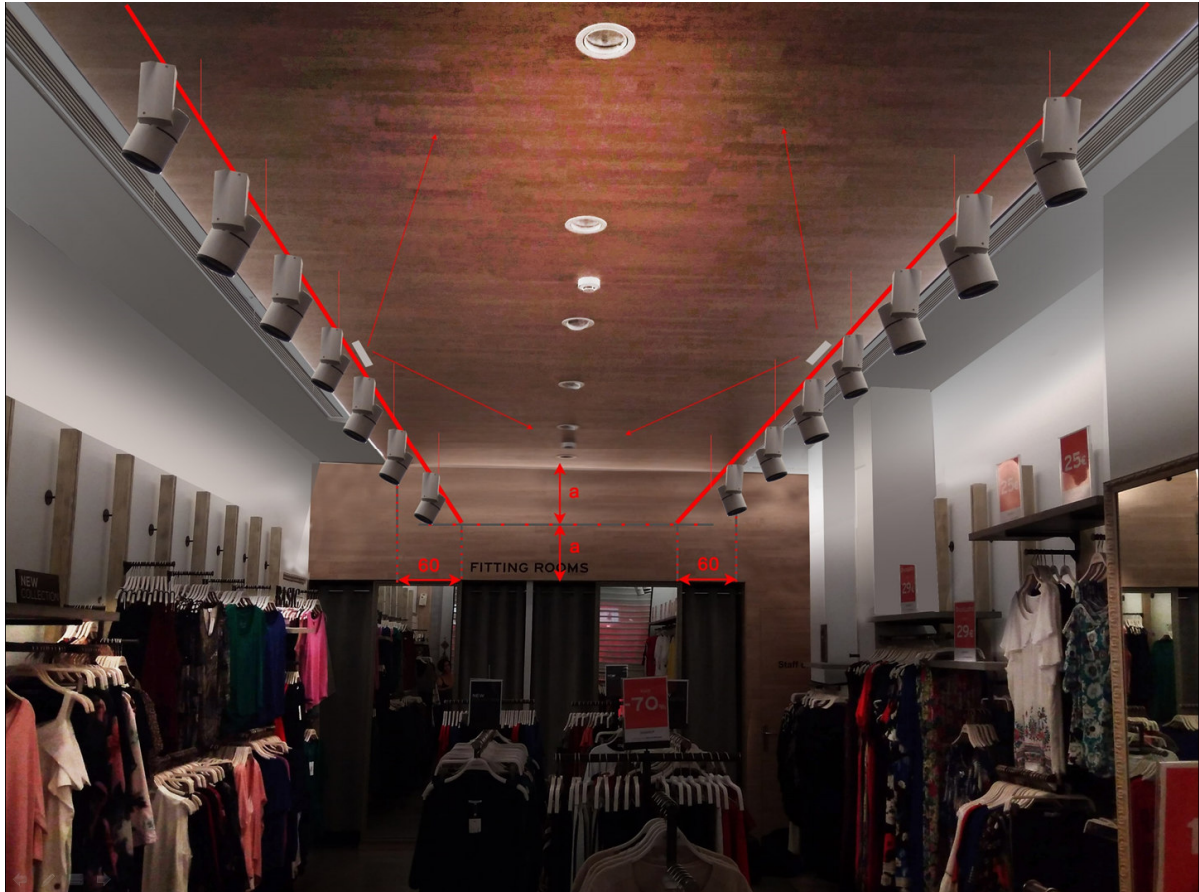
Photo 4: View of the quality of lighting after the renovation
