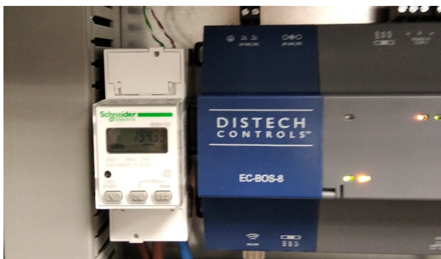
Photo 2: Installed control system and electrical energy measurement system
