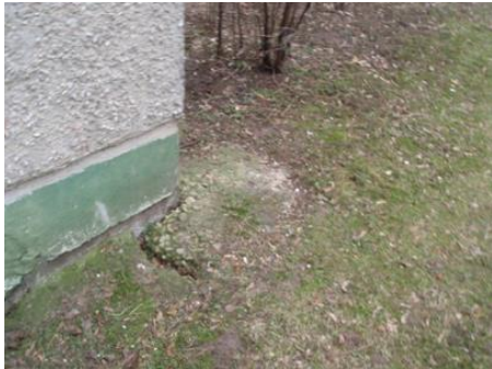
Damaged building plinth
