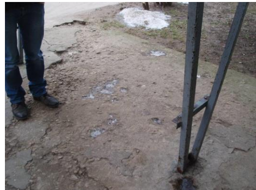
Entrance monolithic concrete damaged
