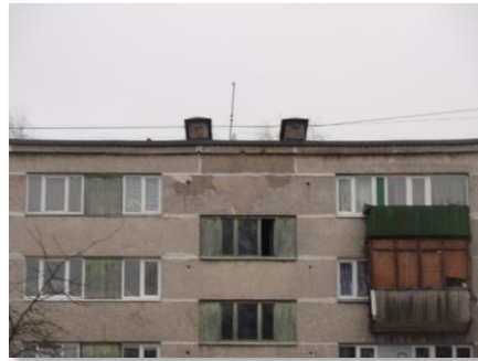
Damaged facade and cap fittings
