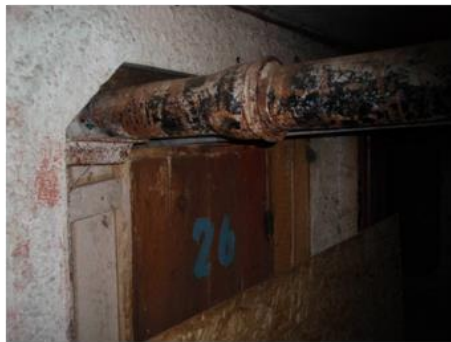
Sewer output from the building
