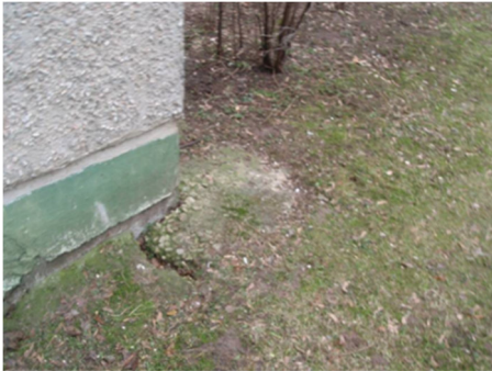
Damaged building plinth
