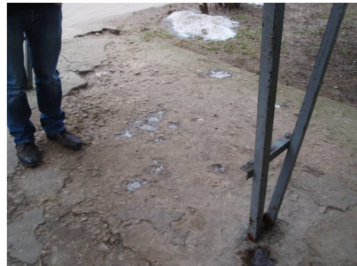
Entrance monolithic concrete damaged
