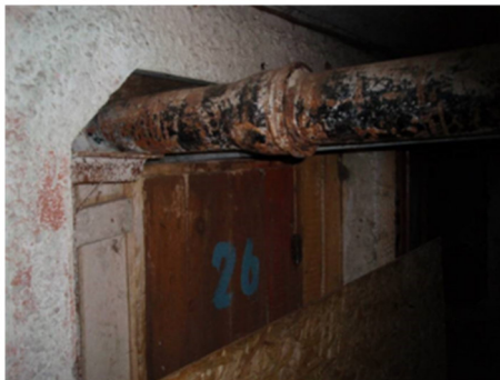
Sewer output from the building
