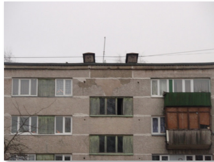
Damaged facade and cap fittings
