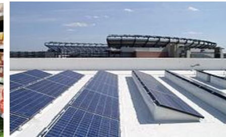
PV for newspaper building
