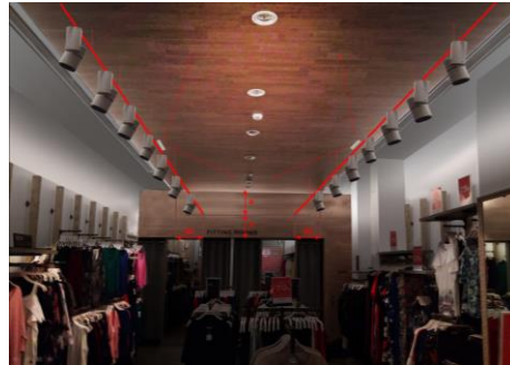
Re-design of the indoor lighting in Greece
